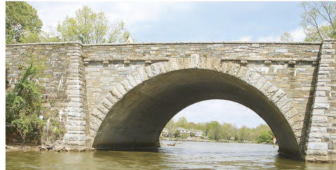
The GW Memorial Parkway's stone bridge over the mouth of Little Hunting Creek.
